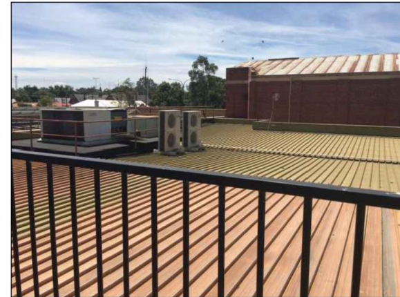
EXISTING GROUND FLOOR ROOF TO BE REMOVED FOR ADDITION AND EQUIPMENTS TO BE RELOCATED
